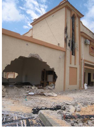
House in Gheiran neighbourhood where pro-Gaddafi forces parked a tank in the living room to conceal it. © Amnesty International
