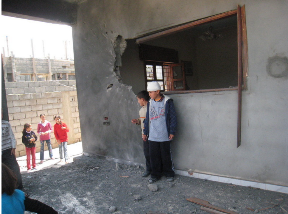
Several residents were injured, including two children, when a mortar struck this house in Gheiran neighbourhood © Amnesty International
